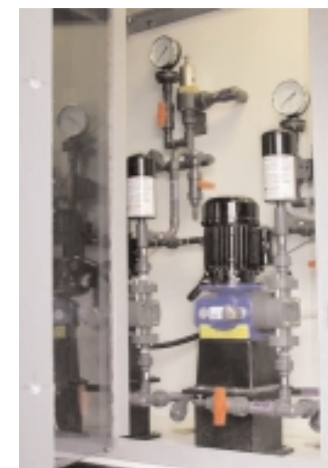
Dosing Pump Compartment
